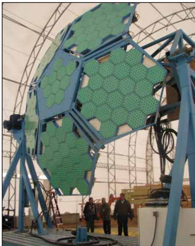
Schriever Air Force Base, Colo. - Workers review the assembled Geodesic Dome Phased Array Antenna Advanced Technology Demonstration. Testing is currently underway and the system is scheduled to be connected to the Air Force Satellite Control Network.
